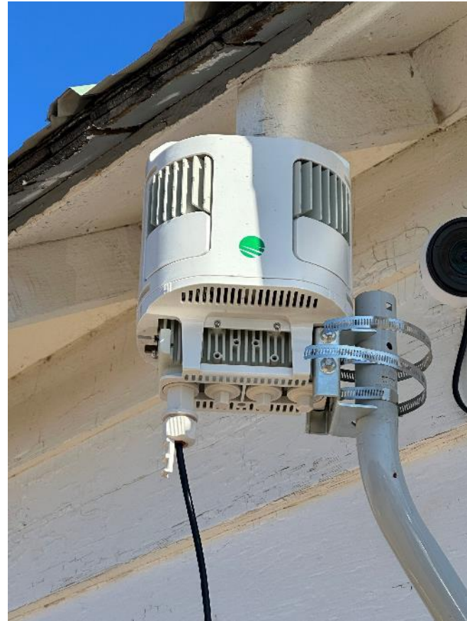
Test Network at Ascent HQ
